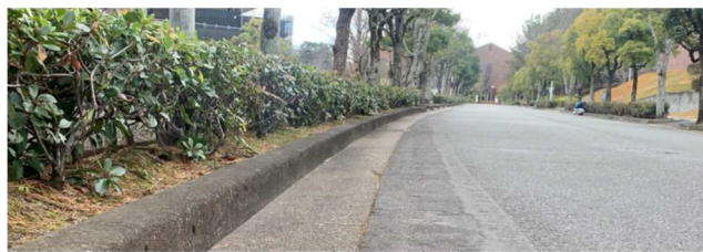
(c) Curbstone. The longitudinal offset from road is 150 mm.
