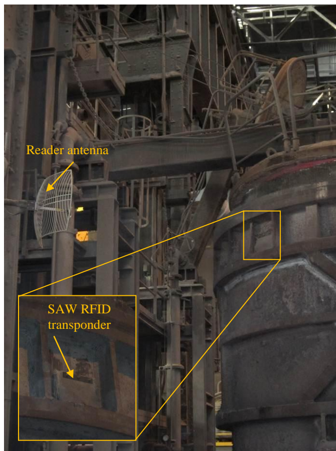
Figure 10. SAW RFID installation on a steel ladle (Georgsmarienhütte, Germany).
