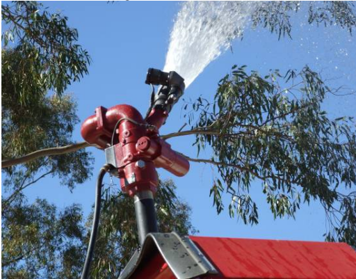
Fig. 1(f) Water Spray Monitor
