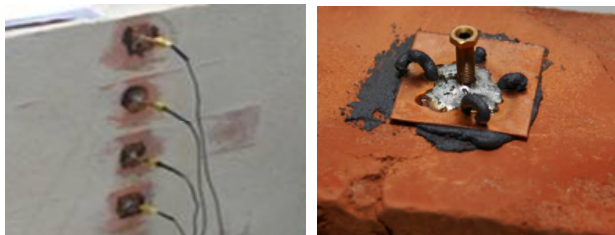
Figure 3. Surface electrodes on the damp brick wall.
