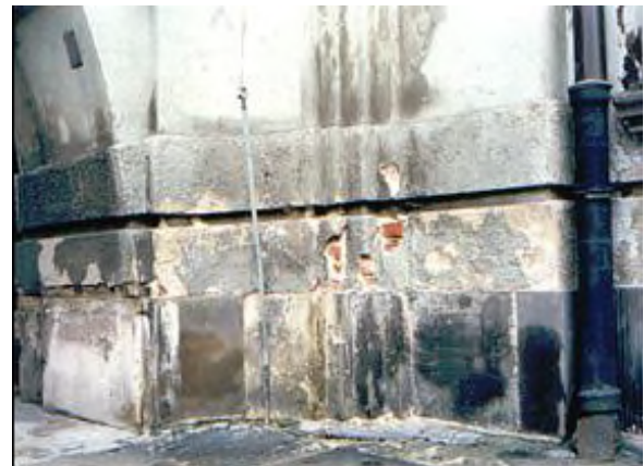
Figure 1. Historical damp wall. Examples of excessively damp brick walls in historical buildings.
